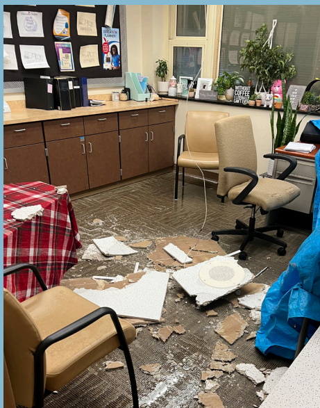
The guidance office was among the most damaged spaces after a sprinkler malfunction flooded the building on Dec. 24.
