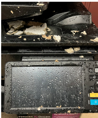
Water damaged the guidance office copier
